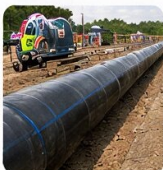
Water Distribution Systems
